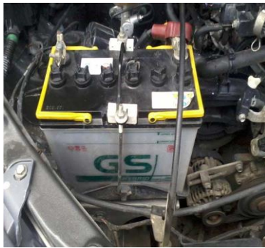
Gambar 4. Lead Acid Battery (BLA)
